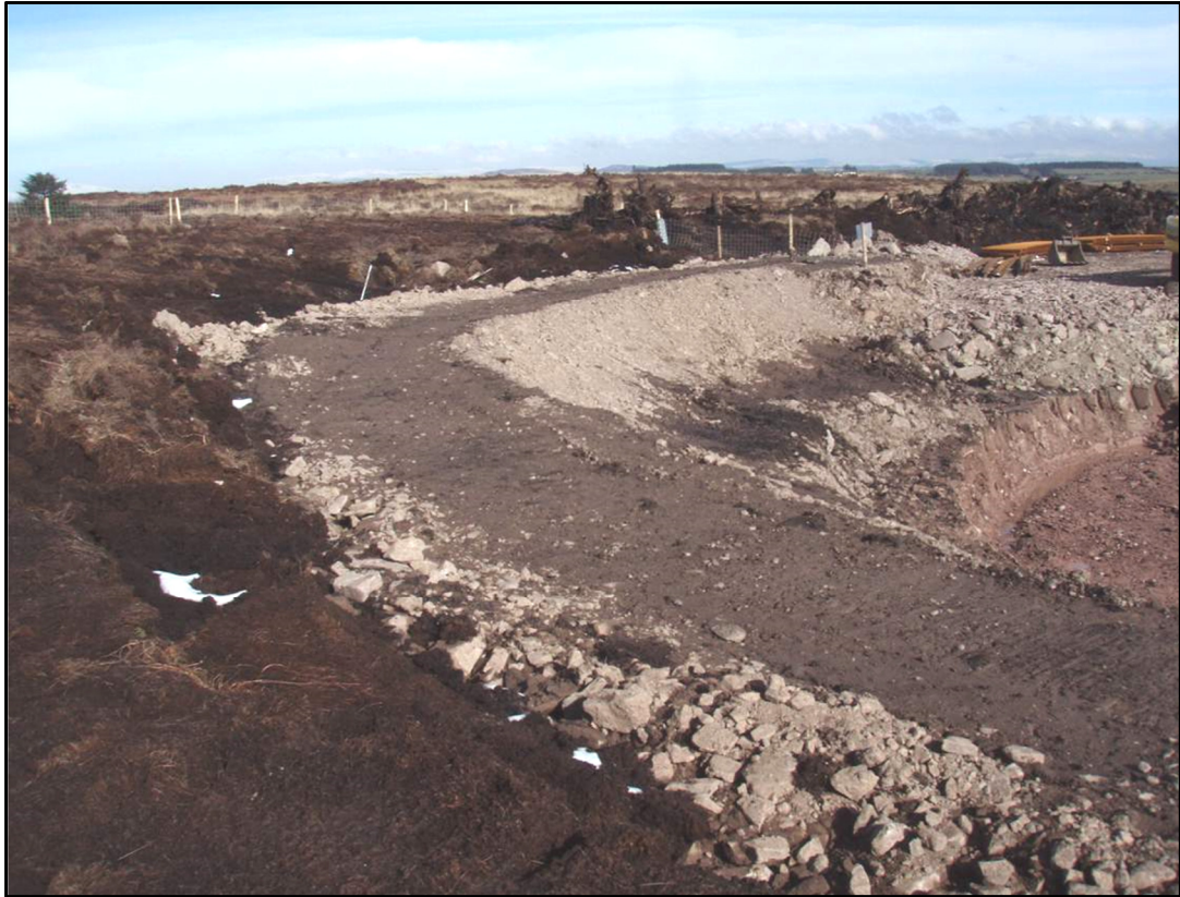
Figure 7-3 Rockfill berm around an area of deep peat on an existing ESB Wind Farm
